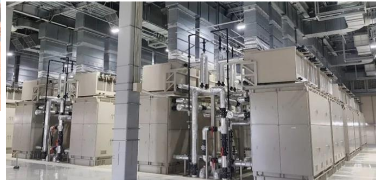
VRFB system - Hokkaido Electric Power Co's power substation in Hokkaido, Japan 60 MWh
