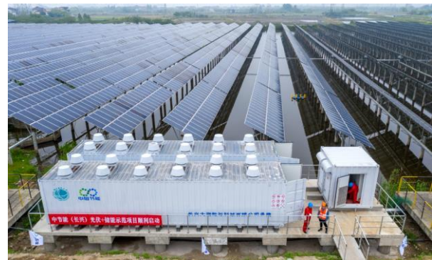
VRFB storing Solar Collection – China (Zhejiang Province)
