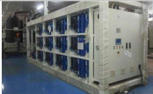
400 MWh VRFB from Pu Neng in Hubei
