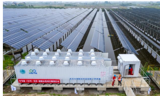
VRFB storing Solar Collection – China (Zhejiang Province)
