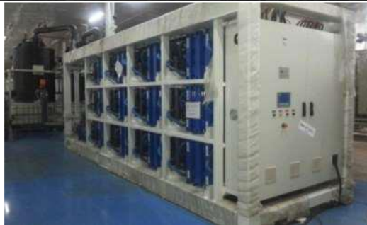
400 MWh VRFB from Pu Neng in Hubei
