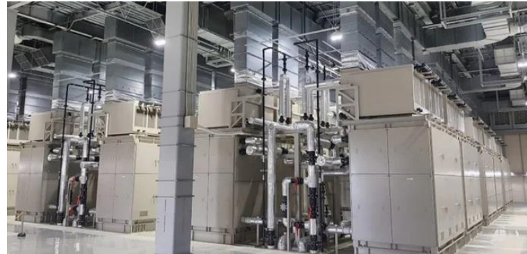
VRFB system - Hokkaido Electric Power Co's power substation in Hokkaido, Japan 60 MWh
