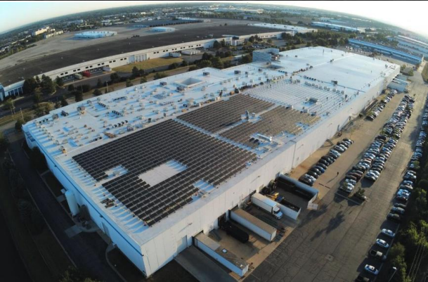
G&W Electric microgrid solution - Illinois, US. – 8MWh
